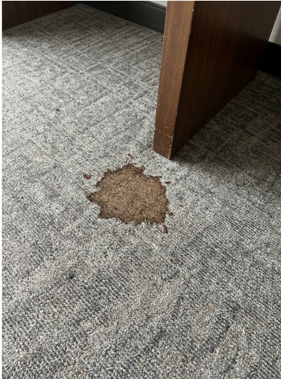
Photo of the defect
