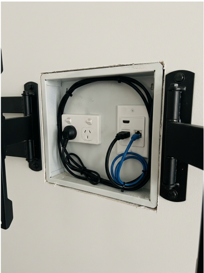
Photos of the back box and connections
