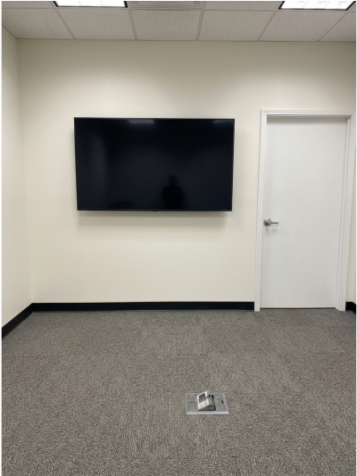
Photos of the installed screen
